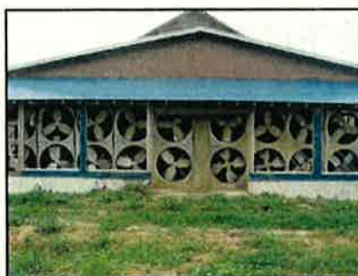
↑牛舎壁面の換気扇
